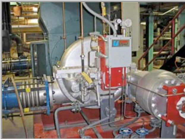
Colorado State University – 801 kW dual turbine system installed, Fort Collins, Colorado
