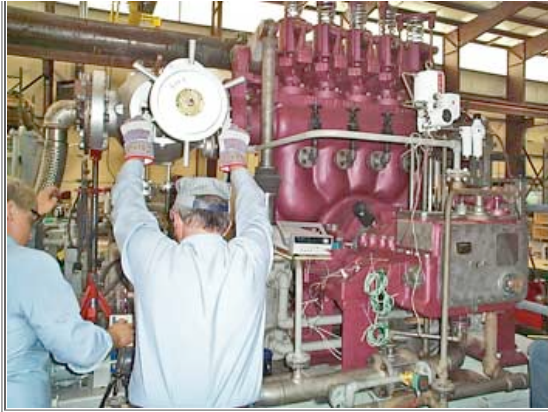
Baltimore Refuse Energy Company – a 4.2 MW turbine generator installed by Turbosteam in Baltimore, Maryland
