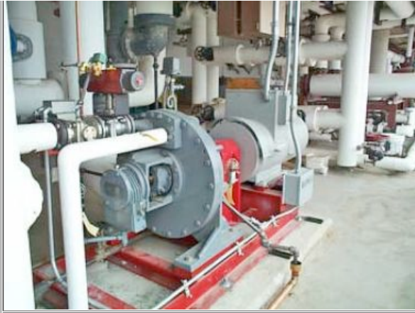
A 50 kW unit at a university in Pittsburgh, Pennsylvania
